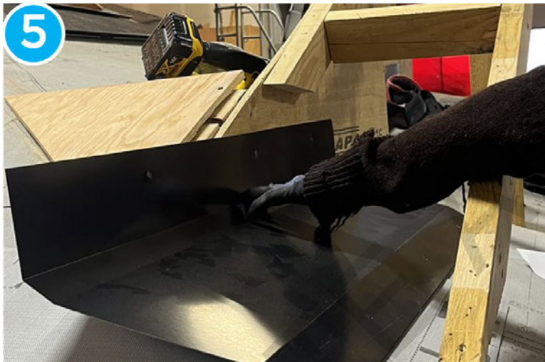
Mark the point where the channel flashing and transition flashing intersect. Then, scribe a line along the decking on the back flange. Draw a line connecting these points (6).
