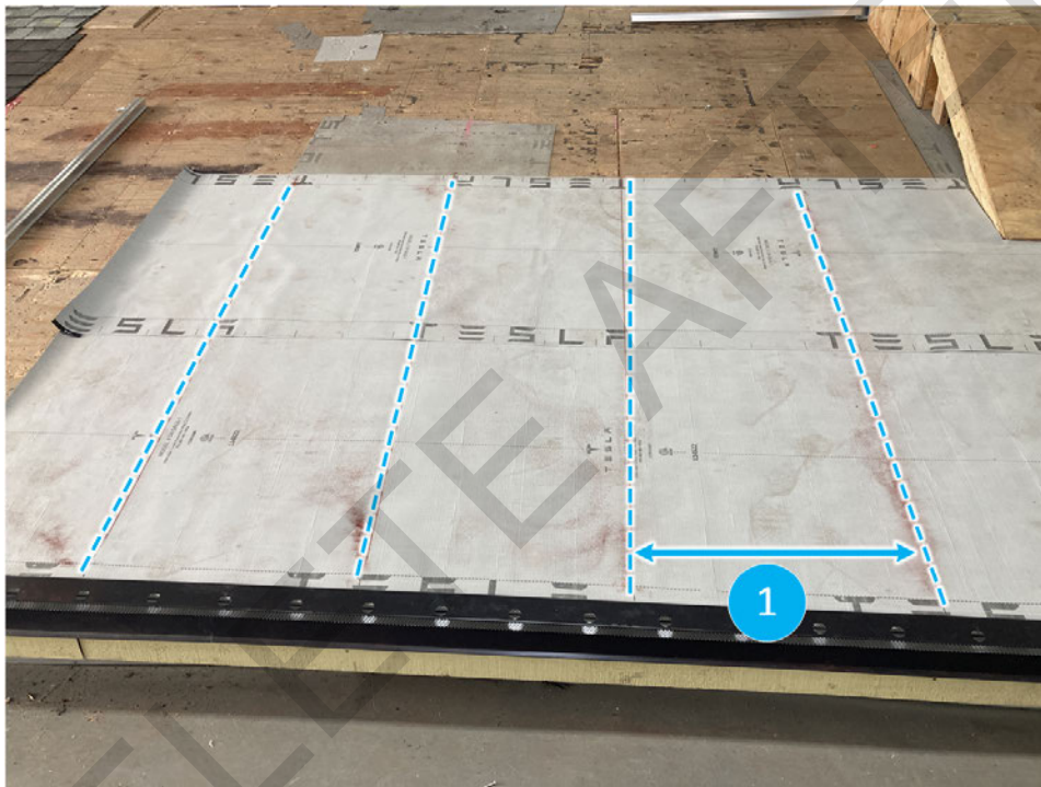
1 - Rafter spacing can vary; always double check with a hammer and if necessary, chalk a line to have a reference of where the rafter location may be.
